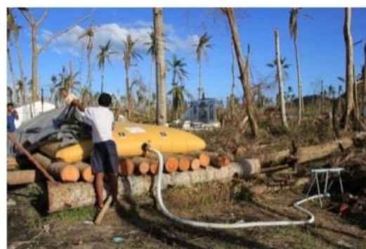
A water tank, filled with 10,000 litres of clean fresh water is installed in Marikina, Leyte (December 2013). Anne Veight/Oxfam
