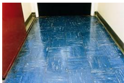
Asbestos containing floor tiles in a corridor
