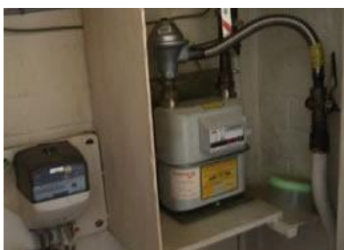
Asbestos panelling around a gas meter
