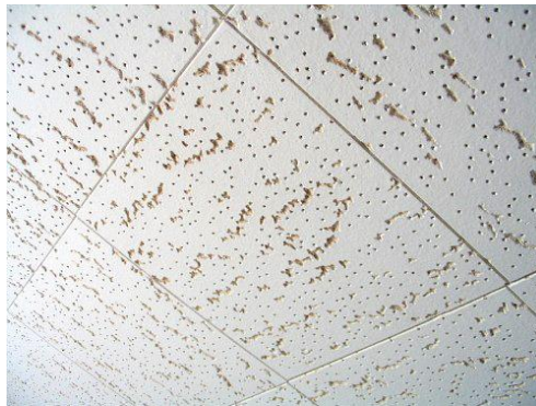
Asbestos containing ceiling tiles
