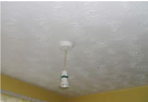
Asbestos textured coating
